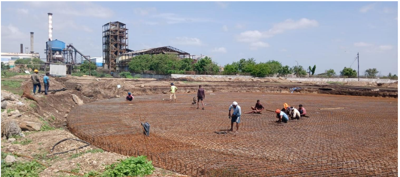
Compressed Bio Gas (CBG) Digester Raft
