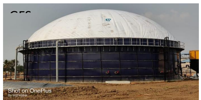
GFS Digester Tank (Completed)
